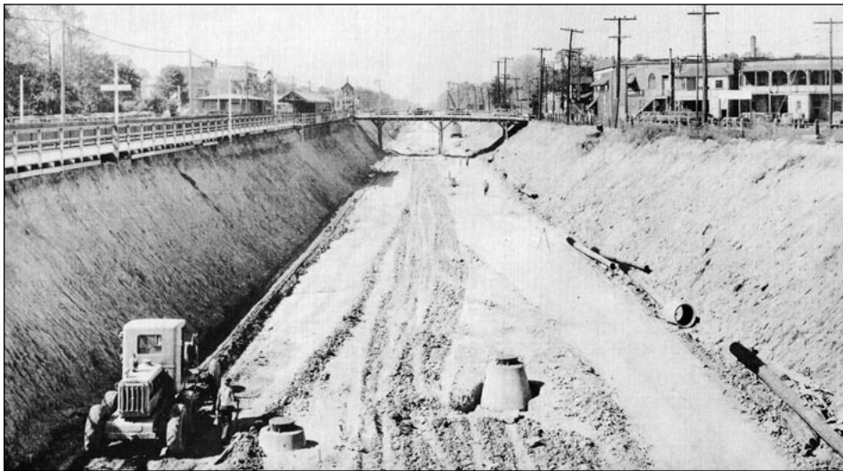
▲ The first grading operation and storm sewers completed—fine grading preliminary to construction of permanent tracks for North Western shown here. Note temporary North Western Elm Street Station facilities at left.— Courtesy of Northwestern University
