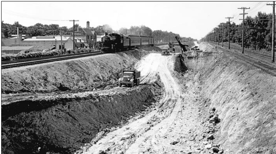
▲ Pine Street is two blocks north of Elm Street. Winnetka is known for its series of streets named after classifications of trees. On August 10, 1939, we are looking north at the digging of the first trench. A southbound suburban train is approaching. We clearly see that there is now a single pole line between North Shore's two main tracks and there is only a single bracket arm on the C&NW pole line as a result of the new system for Western Union.— Courtesy of Winnetka Historical Society
