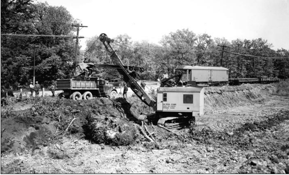
◀ Gage Street is in Hubbard Woods. Digging of the first trench is underway on May 25, 1939. Note the Merchandise Dispatch car now in work service coupled to two flat cars. Please note in the prior photo how North Shore's two main tracks are between the pole lines. In this photo it appears that pole line has been moved to between the two main tracks.— Courtesy of Winnetka Historical Society
