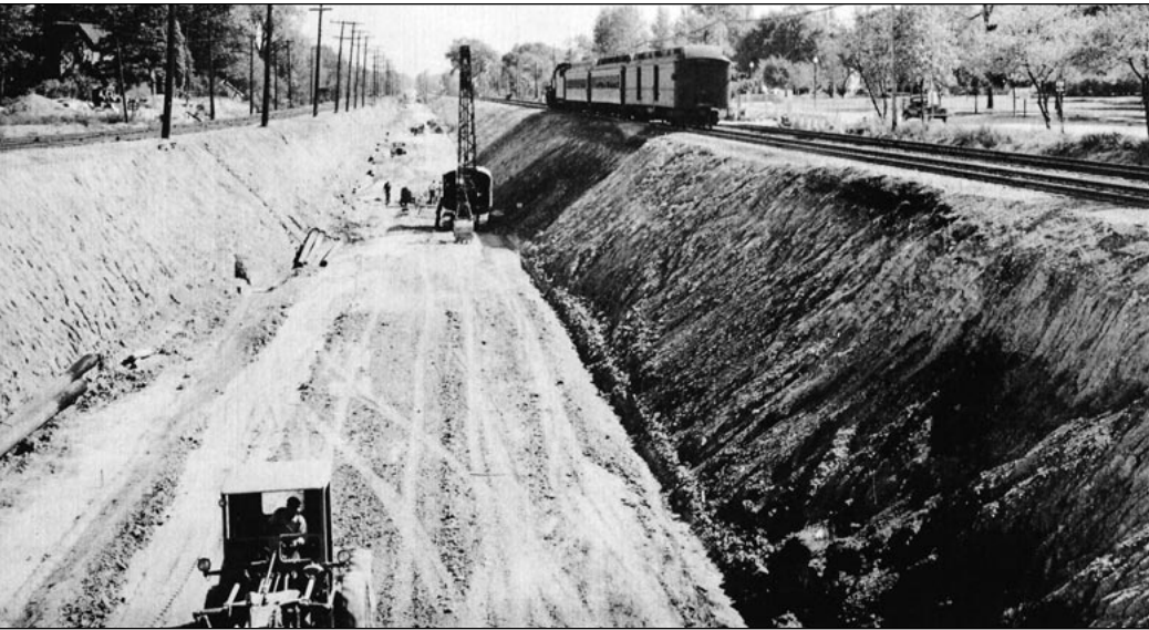
◄ As a preliminary to the first grading operation—tracks and three stations were built for the temporary operation of the Chicago & North Western Railway Company along the westerly side at the right-of-way. These facilities—contracts I and II—were completed early in 1939 at a cost of $342,000 by C.E. Carson & Co. and Deckert and McDowell, Contractors. This view shows the first cut completed in the space formerly occupied by the North Western tracks between the temporary tracks on the right and the North Shore tracks at the left.— Courtesy of Northwestern University
