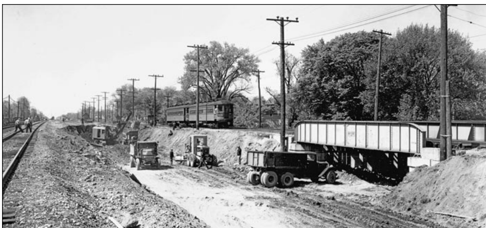
▲ Willow Road originally went under C&NW and the North Shore. On May 19, 1939, the C&NW bridge has been removed and filled in and the trench for the permanent C&NW track that was used temporarily by the North Shore is being leveled to the new gradient. A two-car North Shore train is approaching their bridge over Willow Road on their original alignment.— Courtesy of Winnetka Historical Society
