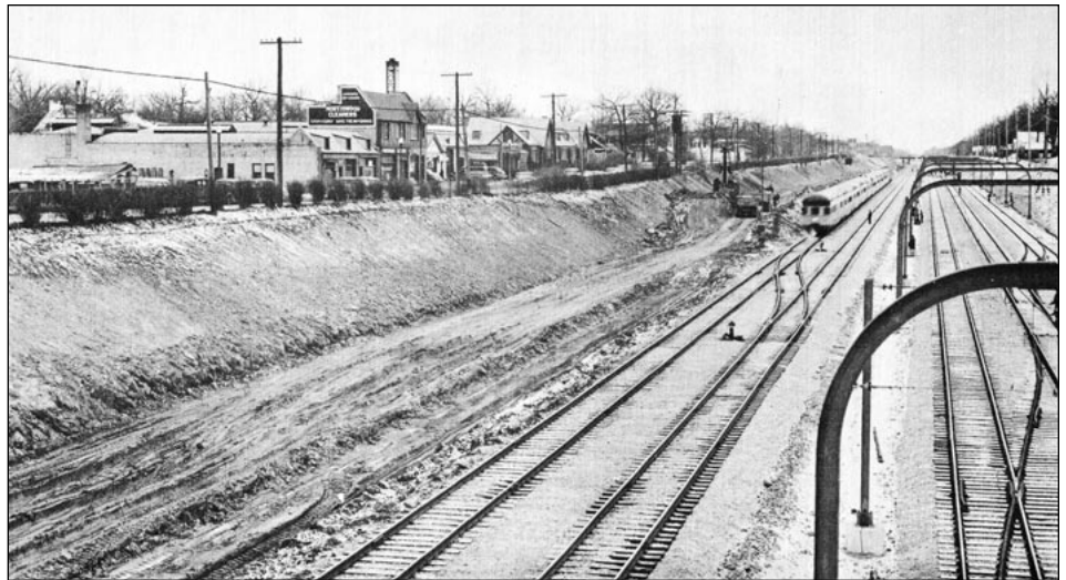
▲ We are looking north from Pine Street at the Pine Street crossovers. C&NW started using its new main lines in May 1941. The third North Shore track at the right is the El Dorado-Elm Siding. What was built at the left in 1941 as a team track is now used by Metra to reverse trains that only operate between Chicago and Winnetka. In the distance is the new streamlined 400 to the Twin Cities. The streamlined 400 was on display at C&NW's Chicago Passenger Terminal next to its heavyweight predecessor on September 18, 1939. The new equipment entered revenue service shortly thereafter.— Courtesy of Northwestern University
